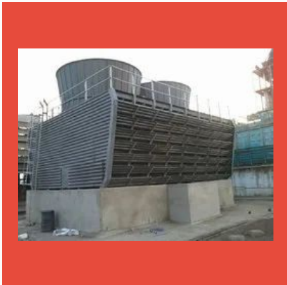
Cross Flow Cooling Tower
