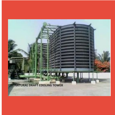
Natural Draft Cooling Towers
