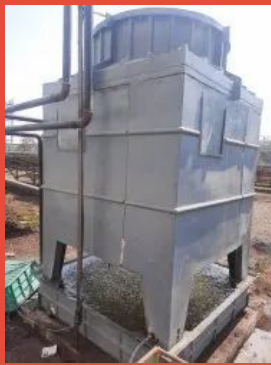
Water Cooling Tower
