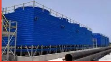
Pul FRP Cooling Tower Multiple Cells
