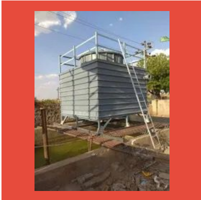
Forced Draft Cooling Tower
